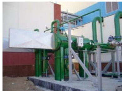
24" / DN 600 FTAF Filter seawater cooling
