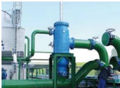
24" / DN 600 FTAF Filter Bioethanol plant
