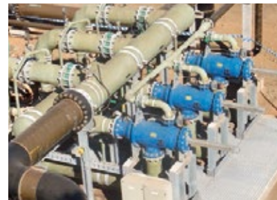
3 x 16" / DN 400 FTAF Filter desalinisation
